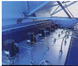
Clean wiring and sleek design characterize the interior as well as the exterior of the 1700EXL
